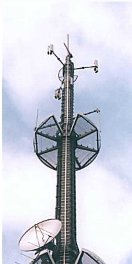
Mast with 6 sectors
